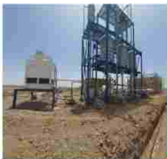
Leachate Treatment system
