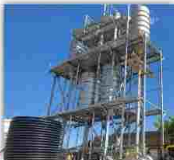
wastewater Treatment system
